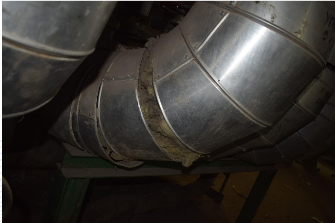
Pipeline damage in a Greek factory.
