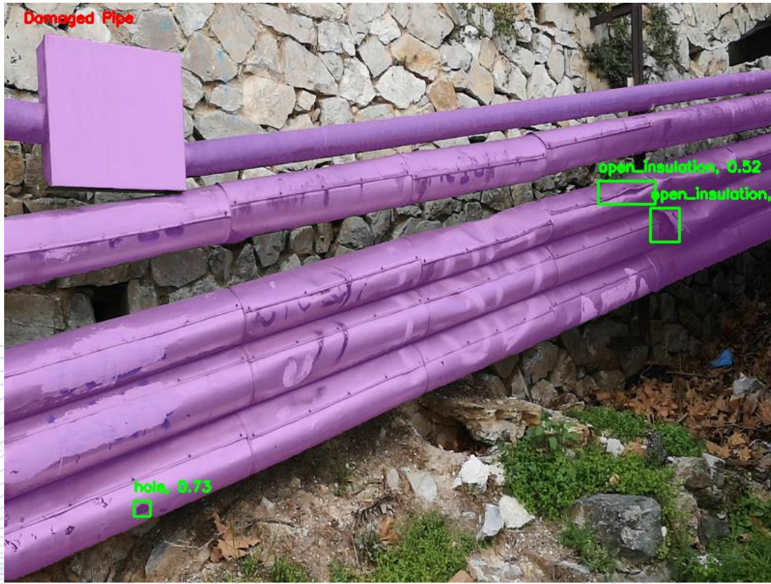
Overall pipeline damage detection and visualization.
