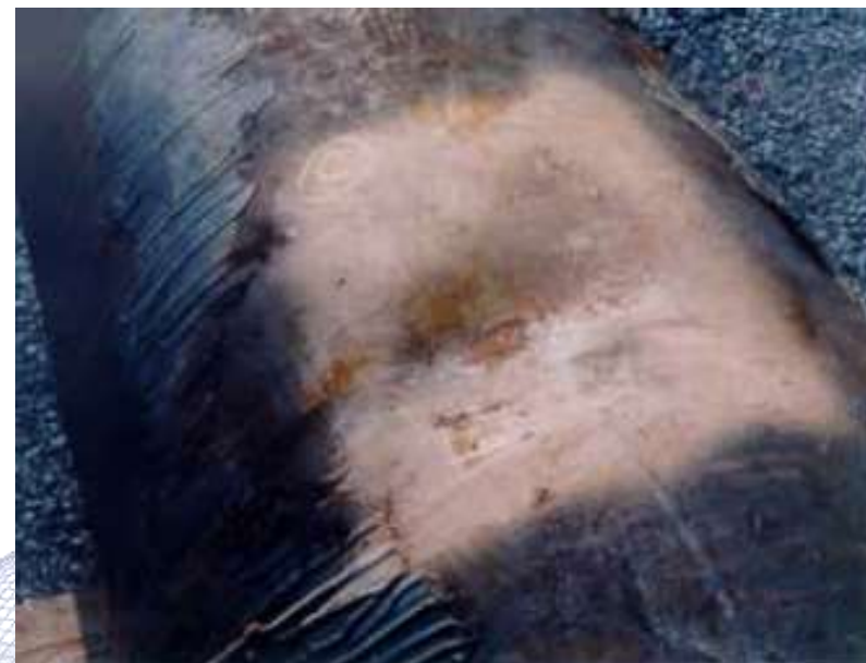
Mechanical failure [SIN2019].
