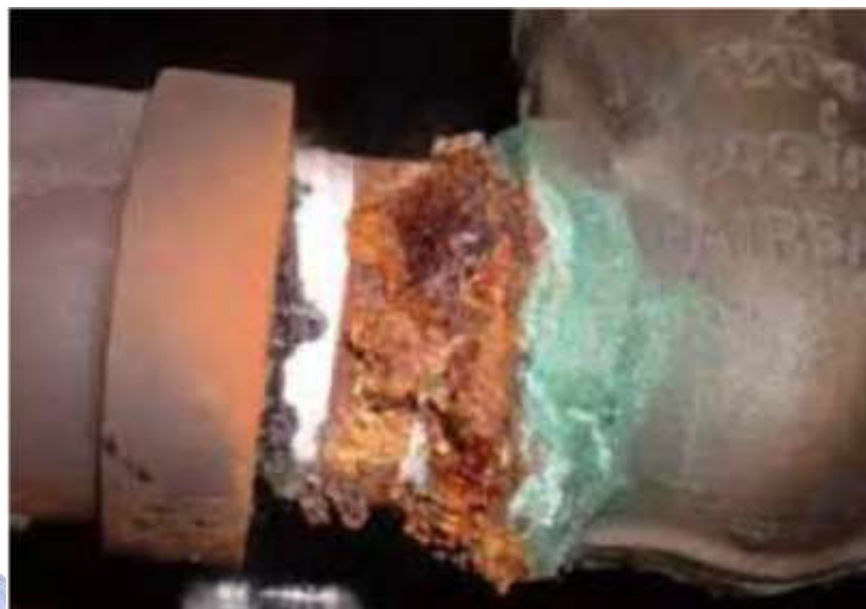
Corrosion damage [SIN2019].
