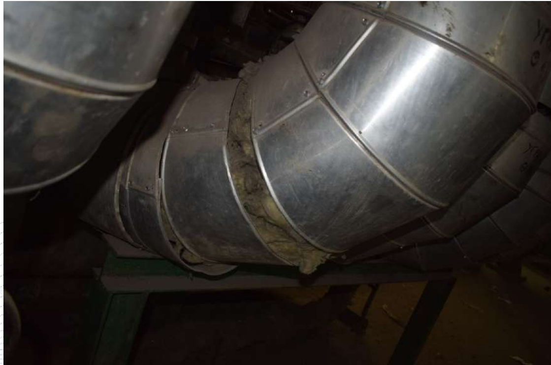
Pipe damage in a Greek factory.
