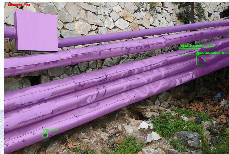
(b) DNN results for pipe segmentation and damage detection.
