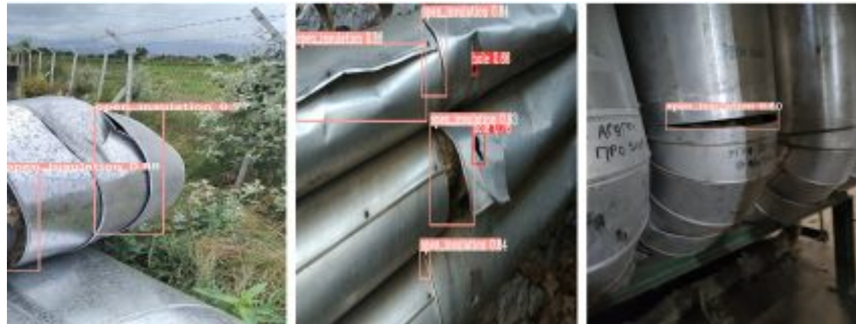
Fig. 5: Inference of YOLOv6 on images from Greek facilities. ("open insulation" damage - pink box, "hole" damage - red box).
