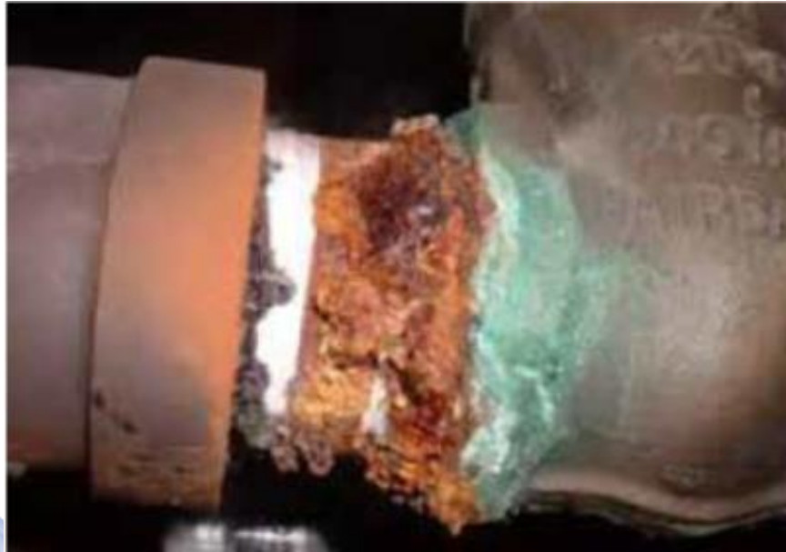
Corrosion damage [SIN2019].
