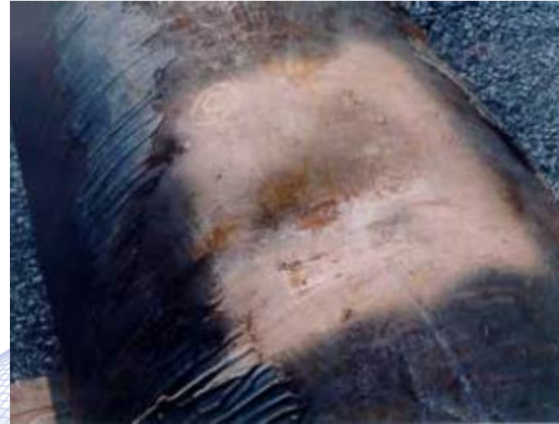
Mechanical failure [SIN2019].
