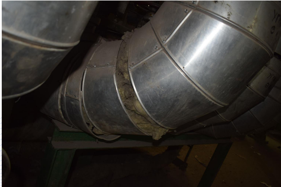
Pipe damage in a Greek factory.
