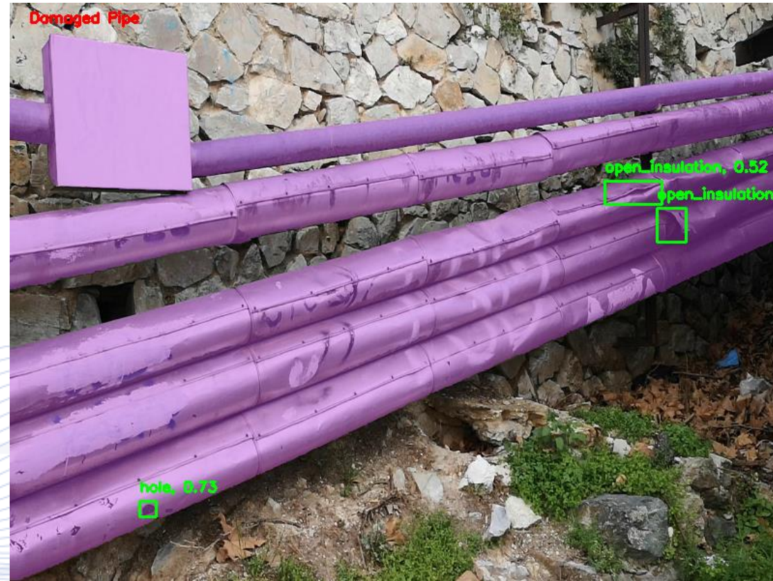
Overall pipe damage detection and visualization.
